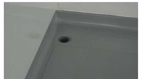
Drain Facility, two drain holes fitted to front of floor
